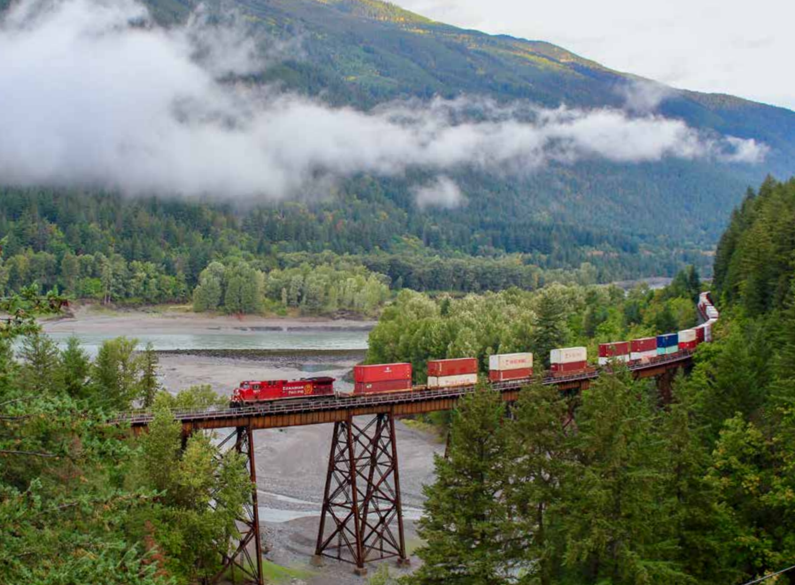
Canadian Pacific Kansas City intermodal train No. 149 from Bensenville, Ill., to the Roberts Bank, B.C., terminal, crosses the Anderson River trestle 2 miles west of Boston Bar on Sept. 26, 2023. Three photos, Bill Stephens
