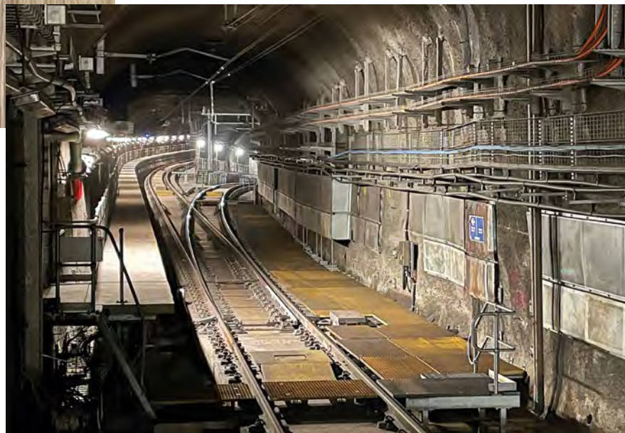
Left and below: Two views looking west from platforms 5 and 6 at Epping on Thursday 2 February 2023. The downhill tracks are the Metro mainlines to Tallawong, while the tracks angled upgrade together form the now unused dive, leading to the above ground Sydney Trains network. Although the two networks share track gauge and overhead power supply compatibility, the signalling and safe working systems cannot integrate, and so it is unlikely these relatively new rails will ever be used again.
