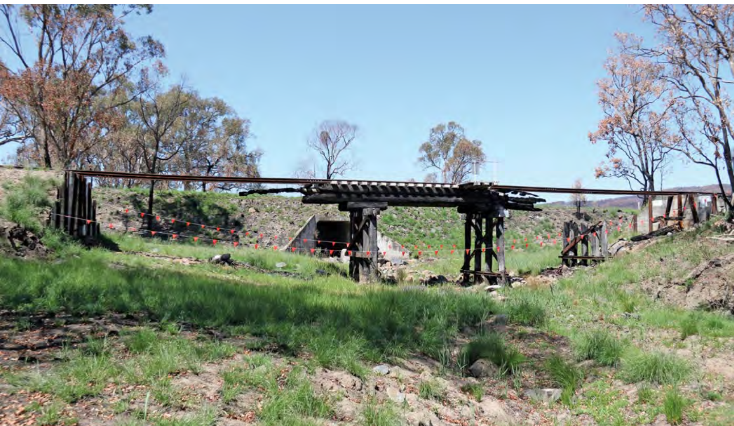
Below: Typical of the damage inflicted by the fire is the condition of this bridge over Accommodation Creek, adjacent to the New England highway, between Bald Mountain and Wyberba, seen on Thursday 7 December 2023. John Hoyle
