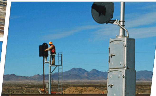
BELOW: As part of UP's double-tracking of the Sunset Route, a signalman sets up a newly installed tri-light signal at Luzena, Ariz., in January 2001. The worker has climbed a ladder to the "basket" to perform his work, as opposed to opening cabinets at ground level, such as on the now out-of-service target signal in the foreground. In either case, given their proximity to the mainline, signal maintainers must be constantly aware of approaching trains via radio, which has been a boon to railroad safety.
