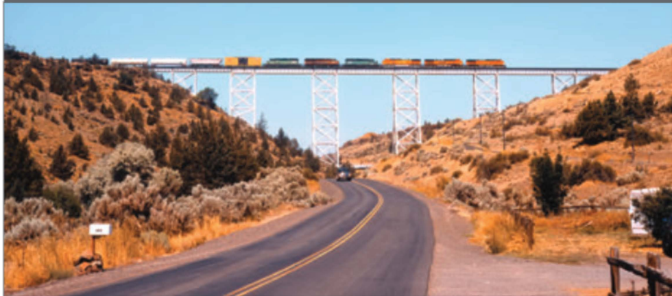
A freight crosses Willow Creek Trestle at Madras, Ore., on August 14, 2006. OTTO M. VONDRAK PHOTO
