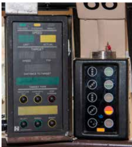
The XITCS display, at left, and UP cab signal display as they were installed in the cab of Amtrak P42 No. 66 during the Dwight-Pontiac 110-mph demonstration. Compare this with the current system shown at right.
