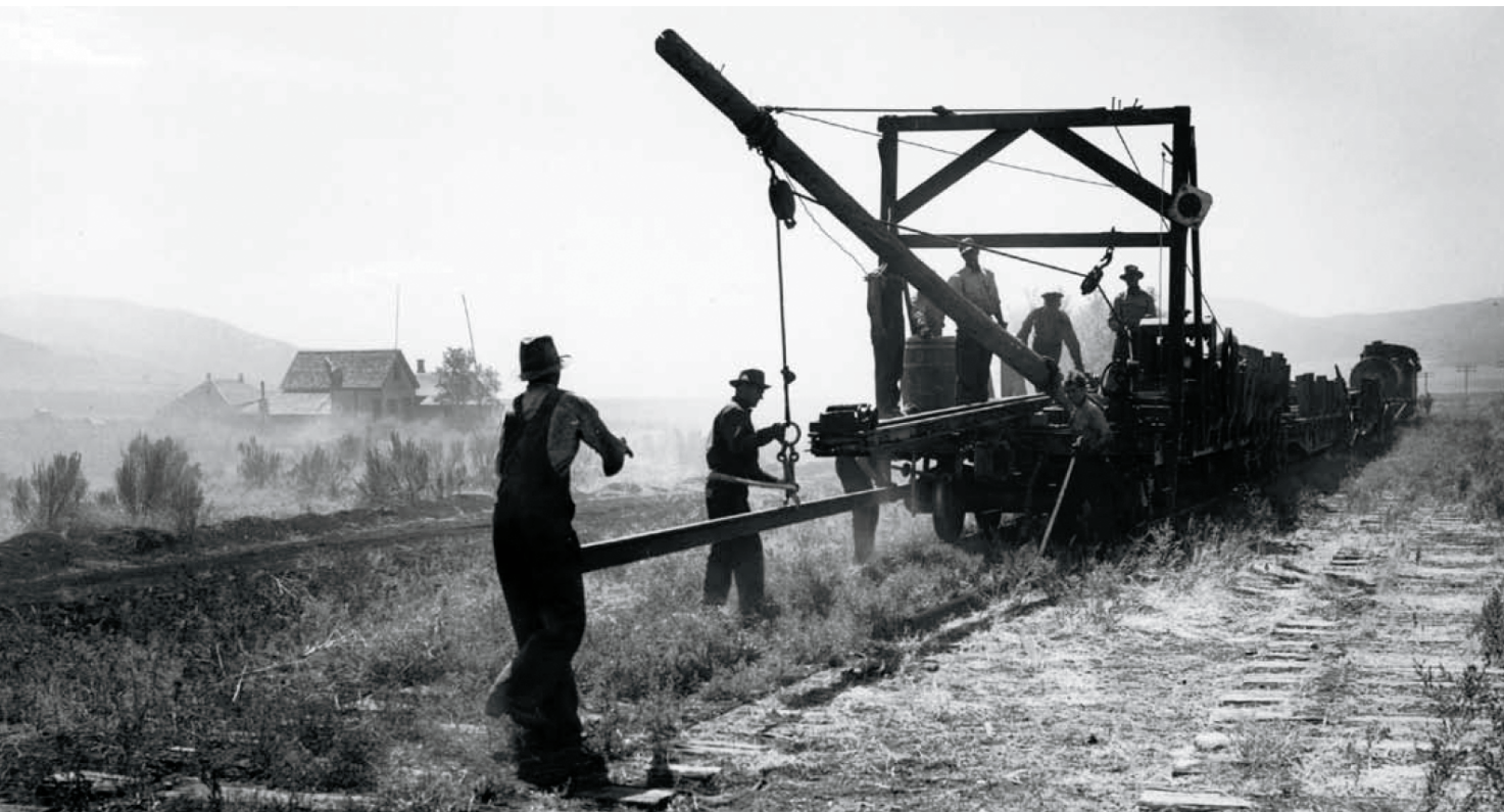
After removal, track material was forwarded to the Clearfield Naval Supply Depot south of Ogden and other military installations for reuse.
