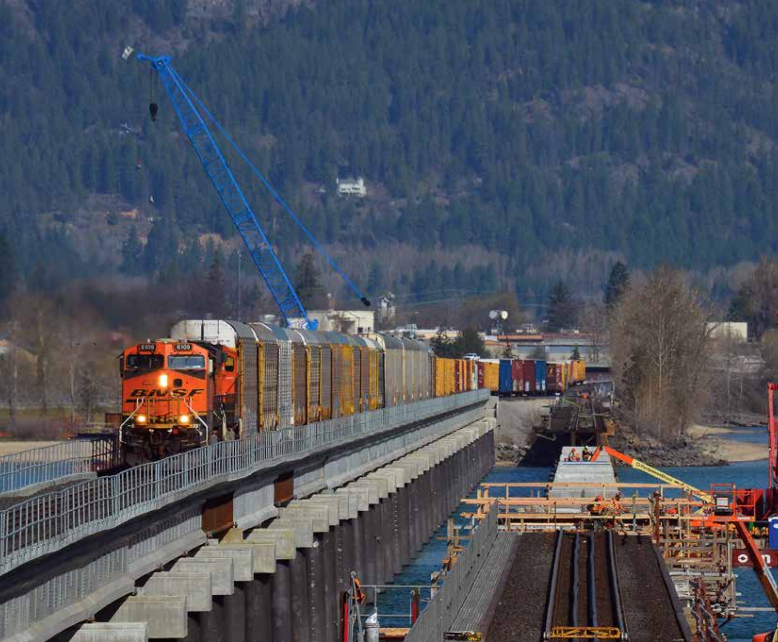
▲ Train H-ALTPAS crosses the new bridge over Lake Pend Oreille, Idaho, on April 29, 2023, while the old bridge undergoes extensive renovation.
