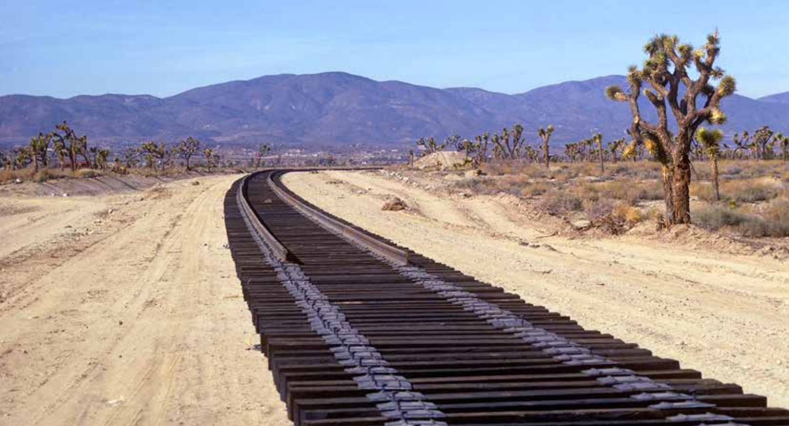
One of the biggest projects during Russell's tenure as SP boss was construction of a 78-mile line between Colton and Palmdale, Calif., that enabled freights to avoid the congested L.A. terminal area. Ties and rails advance across the desert east of Palmdale on February 22, 1967.
