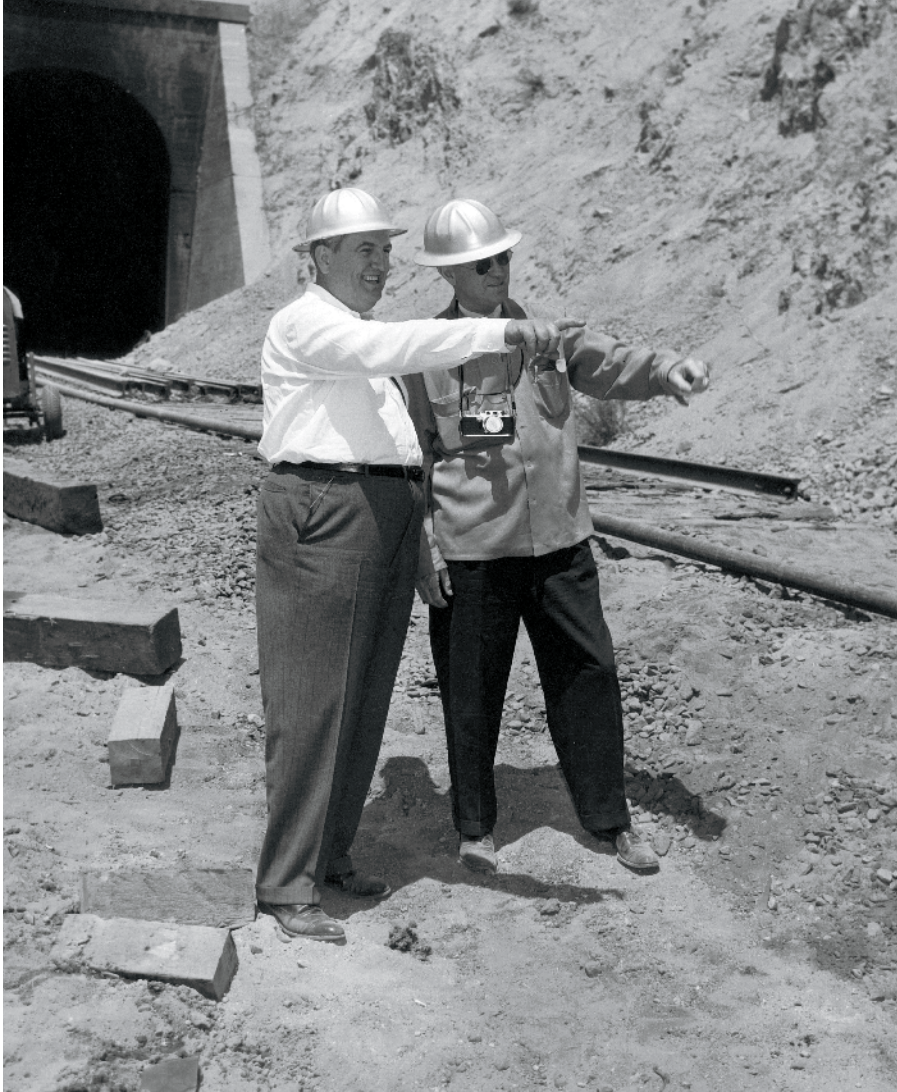
After the July 1952 Tehachapi earthquake, Russell (left) discusses restoration work at Tunnel No. 5 above Bealville with Fred Gurley, president of the Santa Fe, which also used the SP line.
