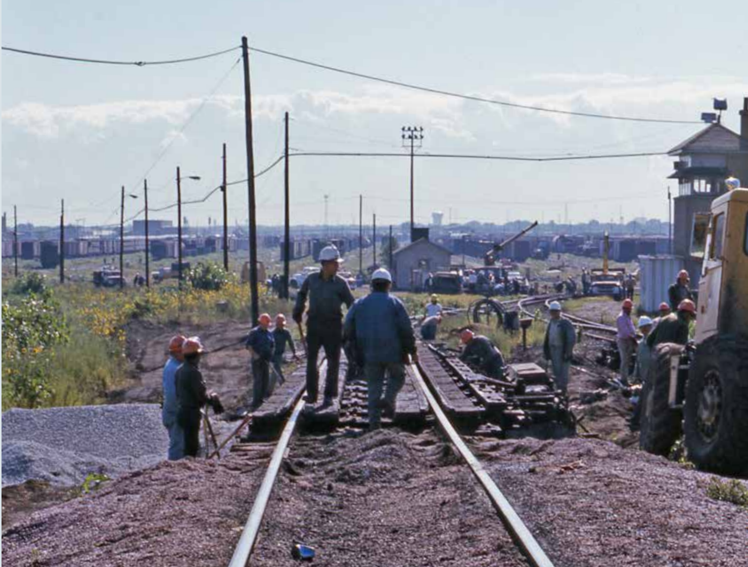
Short-term pain, long-term gain: Engineering Department crews swarm over Proviso's twin humps, shut down for their work, in 1974.
