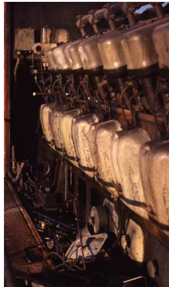
Removal of the engine hood of CP M636 4724 affords easy access for mechanics to remove salvageable parts from the forever stilled 16-cylinder 251 engine.
