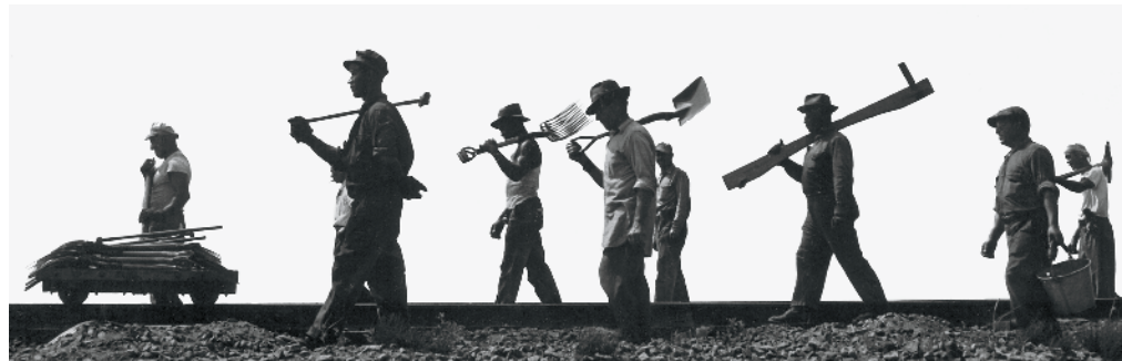
Welded rail and mechanical tampers/liners have ended the need for large crews that maintained track with hand tools. CLASSIC TRAINS collection
