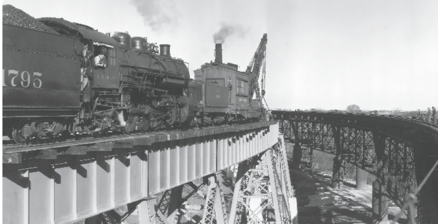
How's this scene of men and machines on the high steel for a scary Halloween treat? On October 31, 1934, Illinois Central 2-8-2 1795 carefully pushes steam derrick X15, carrying a deck girder section, toward placement on the new Kentucky-side approach trestle.
