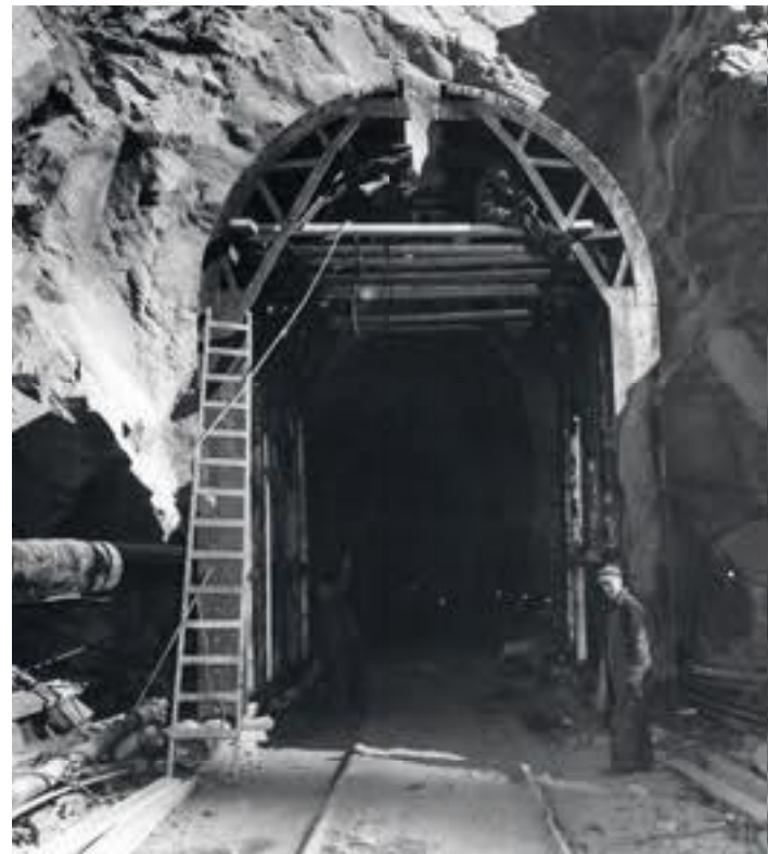
Workers erected a steel arch framework at the western entrance to the fire-damaged 1,570-foot tunnel.
