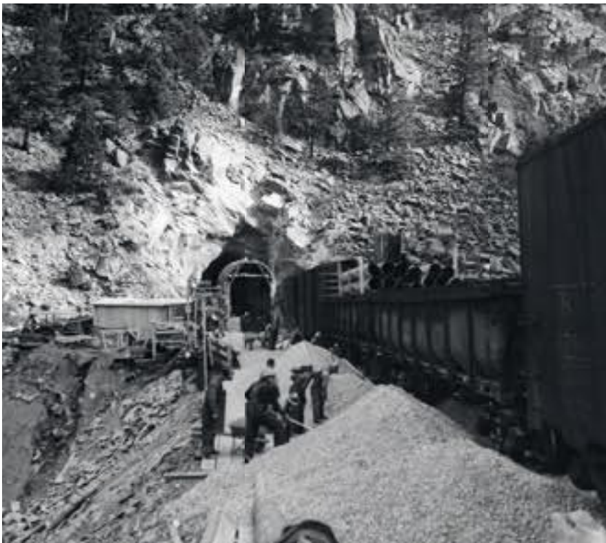
Men are busy shoveling gravel as cars filled with material arrive at Tunnel 10's west portal. Workers from a nearby water tunnel construction project assisted railroad crews.
