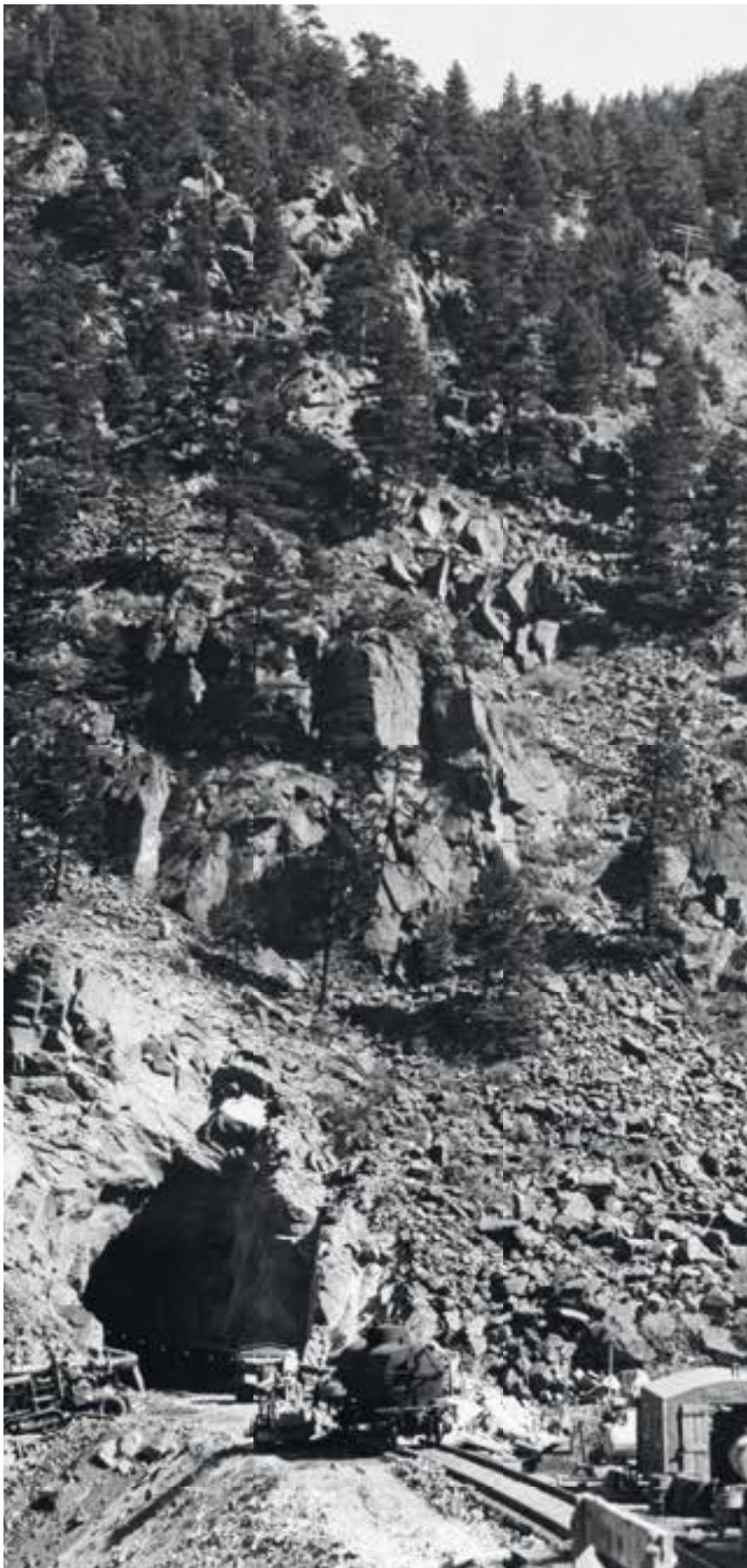
On- and off-track equipment stands outside Tunnel 10's west portal during the early stages of the repair work. Most resources were brought in from the Denver end of the tunnel. Behind the photographer about 300 feet is Tunnel 11.
