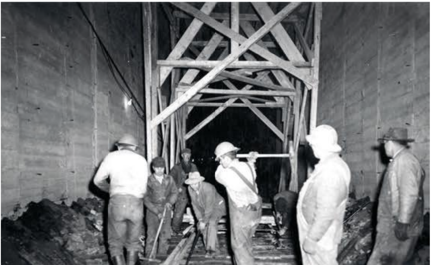
With the concrete lining in place, but some wood framing and rock yet to be removed, track crews spike down new steel inside the tunnel. Thousands of miles from the front lines, these men are doing their part for the war effort.
