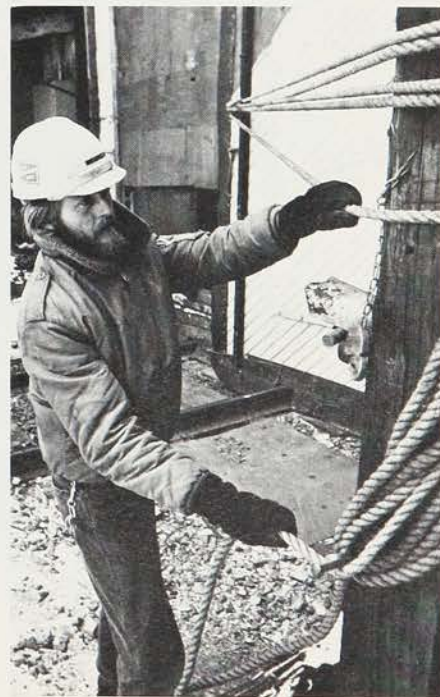
JEFF closes the tunnel doors.
