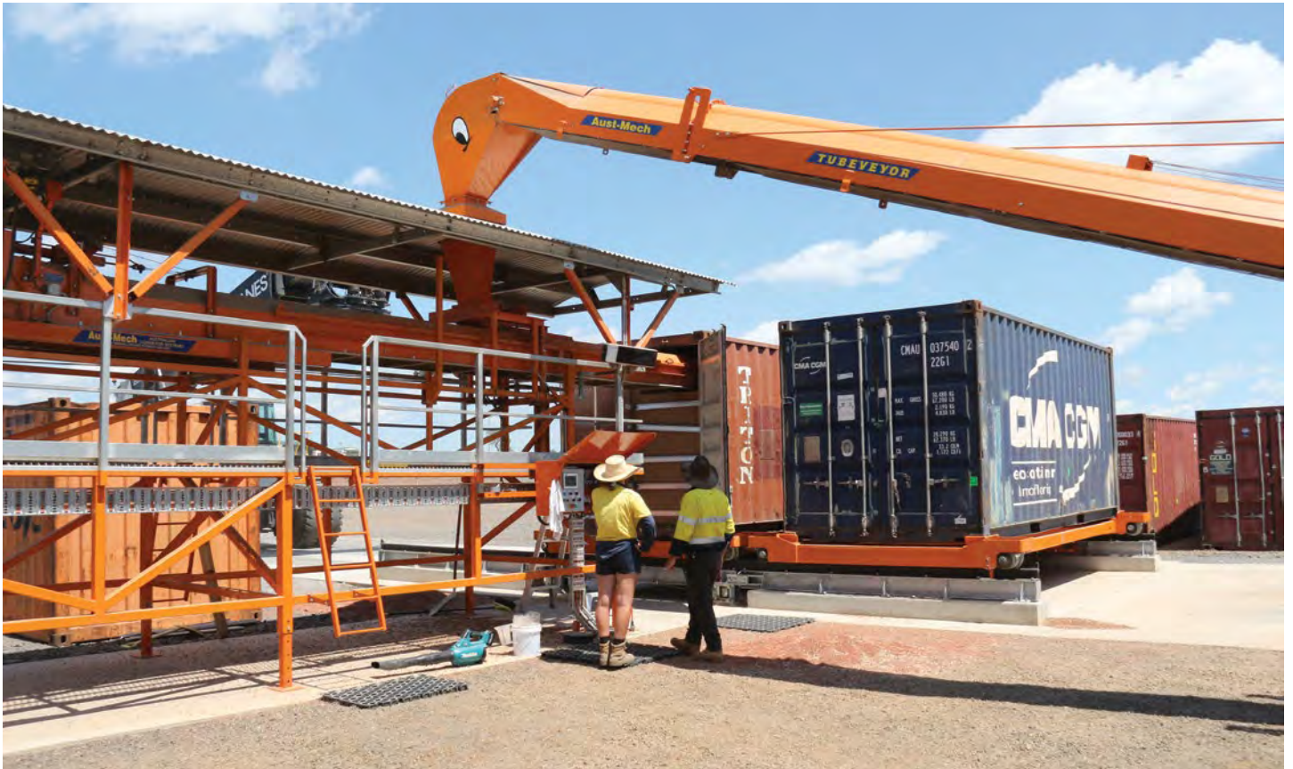
A feature of Seaway's Yamala intermodal terminal is a grain container packing facility seen here in action on Saturday, 18 March. Grain is moved from the company's storage facility to the Aust-Mech "Tubeveyor" seen in this view which drops grain on to a conveyor which transports it in to the horizontal container behind a bulkhead seen here at the end of the container, adjacent to the open right-hand door. Some grain container packing facilities load with containers in the vertical position. A 20-foot container can accommodate 24 to 26 tonnes of grain.
