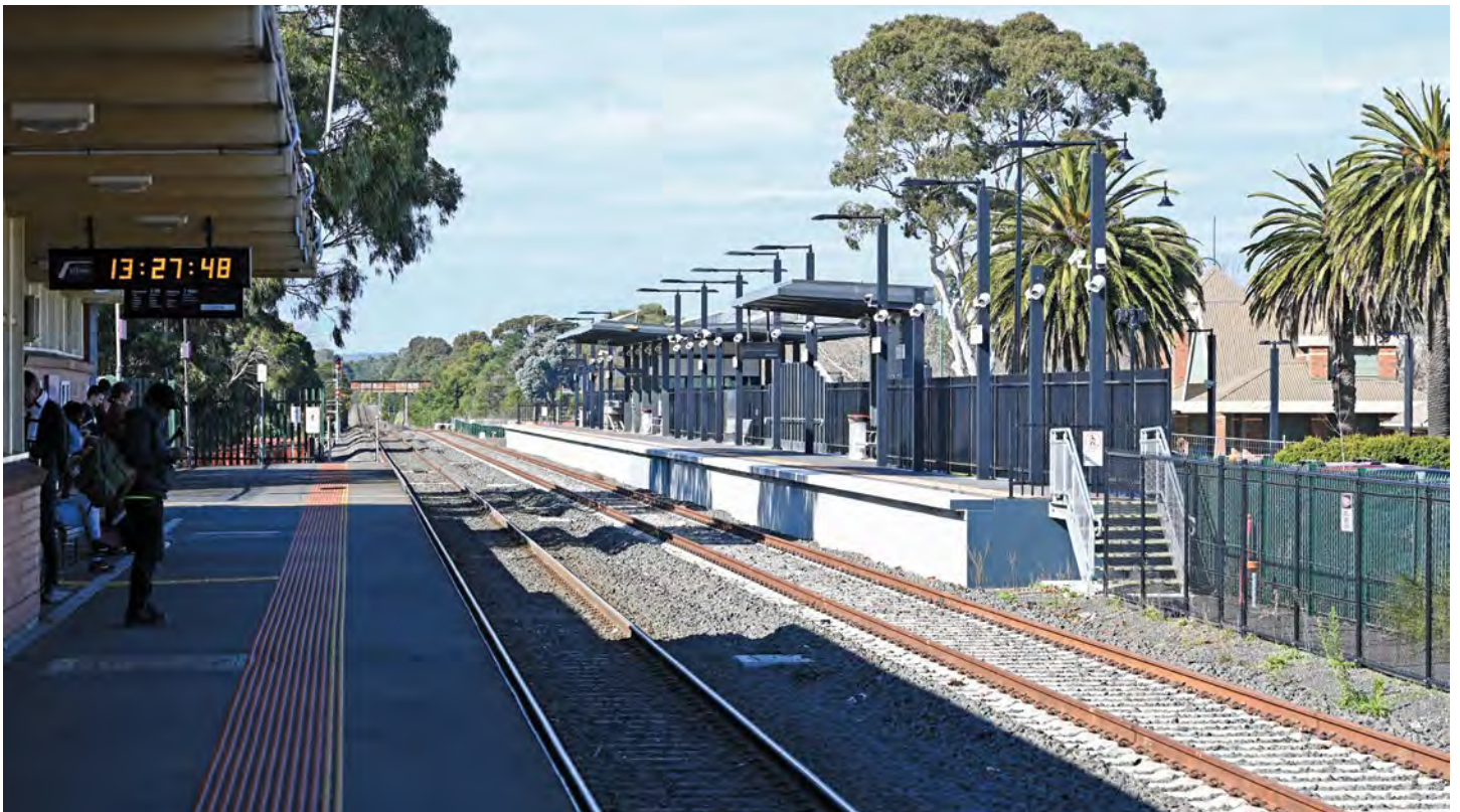
Taken from the existing (single) platform at Morwell, looking in a Down direction, the under-construction second platform is visible, notable for being offset against the existing due to space considerations. The distinctive palm trees here are also seen. The new track will continue east before reverting to single line through to Traralgon. At the time of writing a completion date for this part of the Project has not been announced.
